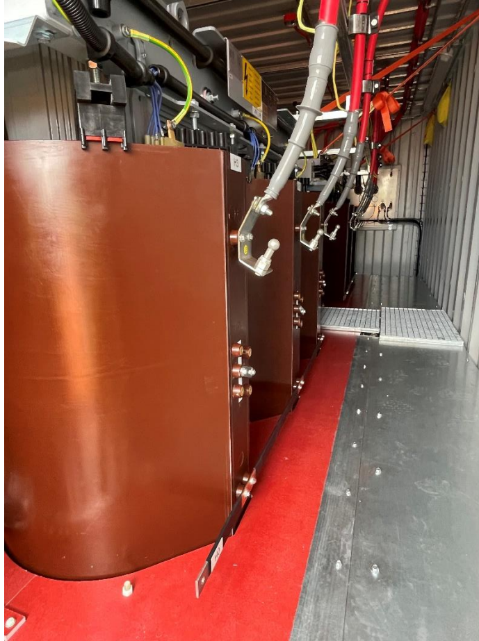
Figure 11- PowerCon Transformer Unit, Matt Creswell
