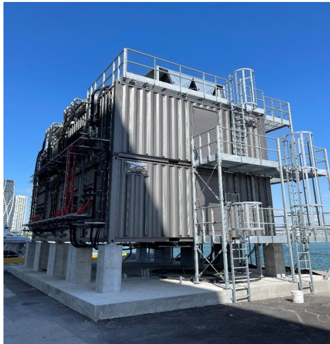
Figure 6- Containerized Transformer Unit, Matt Creswell
