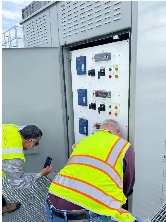
Figure 18- Inspecting spot welds on switch panel door, Matt Creswell
