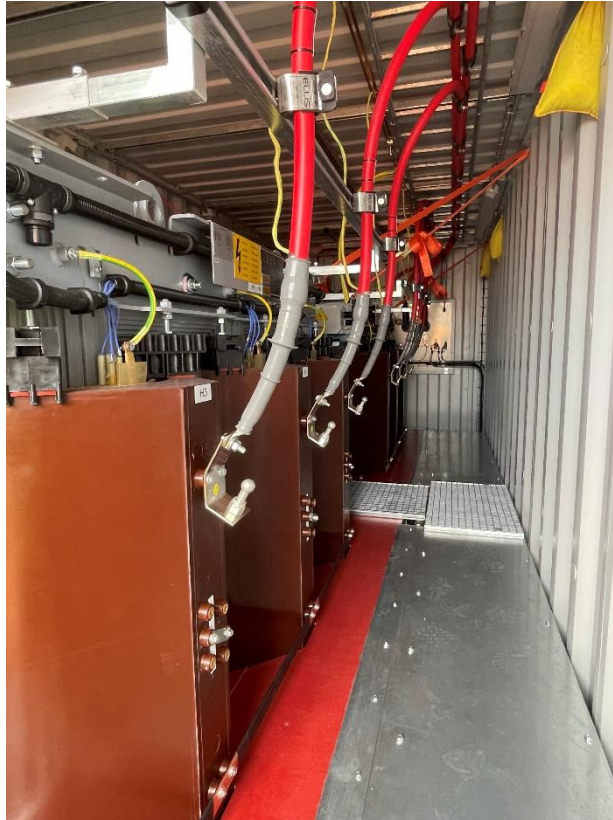
Figure 16- Transformer units, Matt Creswell
