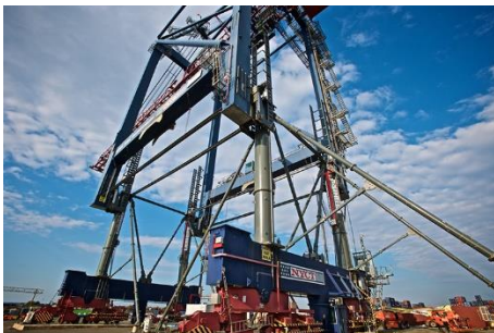
Image_1.jpg The Liebherr STS at Port Liberty receive an 8.6 m lift height increase
