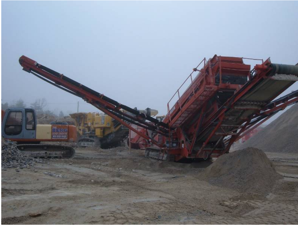
Figure 1. Crusher Used to Produce CCA at the Concrete Plant
